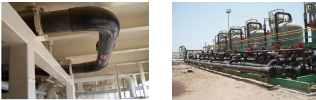
Figure 8. Above-ground pipe system [6]
